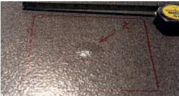
Moisture vapor transmission failure of epoxy quartz system.
